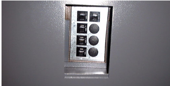
Figure 26: Circuit breaker panel
